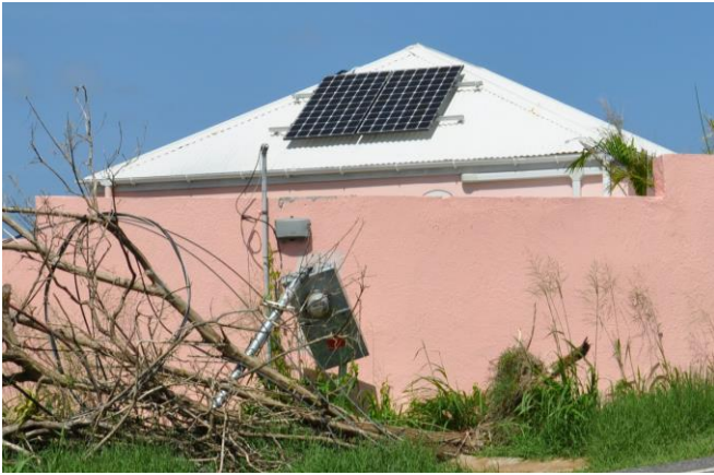
Figure 1. A two-panel array on a residence. The rails were attached with clips that were anchored through corrugated metal roof panels and into the roof structure and/or roof deck. No damage to the PV array was apparent.
