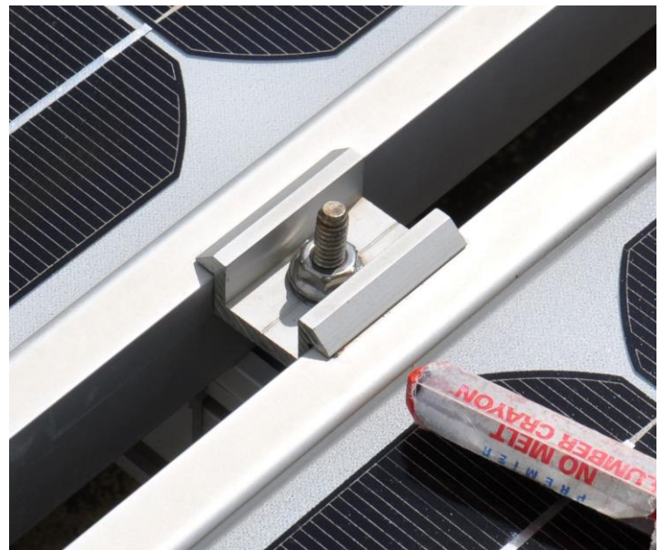
Figure 13. View of a PV panel clip after the 2017 hurricanes. Although there was no apparent loosening of the nut, the bolt could be wobbled with finger pressure. A loose nut such as this is susceptible to further loosening and loss of the clamp's ability to keep the panels in place.
