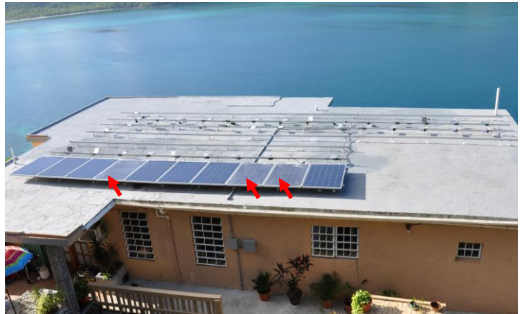
Figure 4. Three of the four rows of panels at this residence were blown off; they detached from the rails. The rails were attached to posts. Three of the remaining ten panels were damaged by wind-borne debris.
