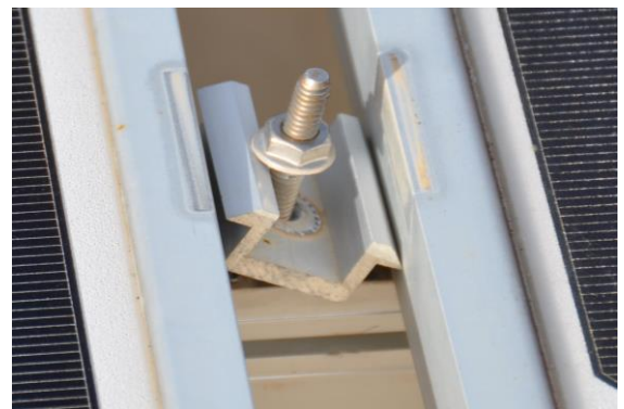
Figure 8. T-bolt with dislodged clamp.
