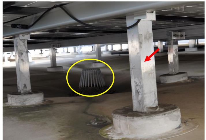
Figure 10. PV panels extended over this roof drain (yellow oval), thereby making it difficult to check for clogging and removal of debris. The red arrow indicates a rail support post.
